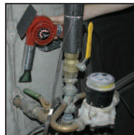
Thaw Frozen Pipes
